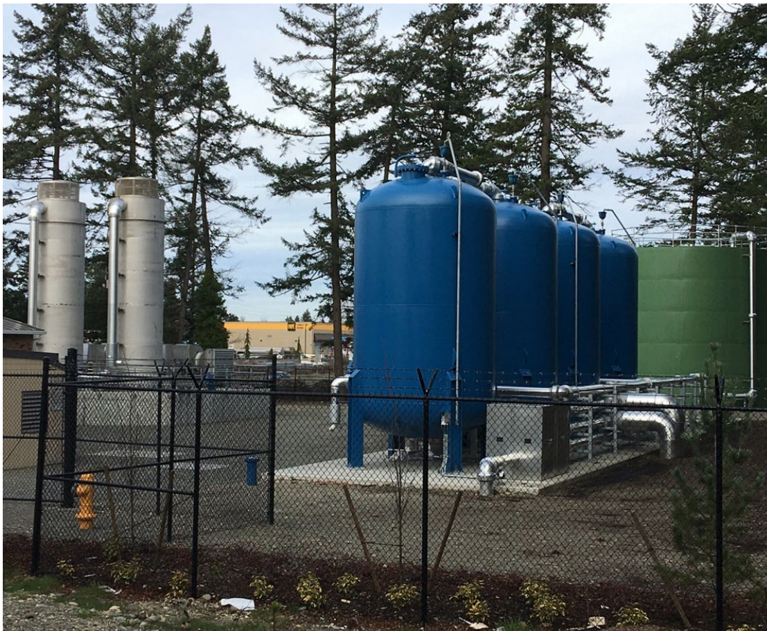
Figure 5: Lakewood Ponders Wells Operating GAC PFAS Treatment System
