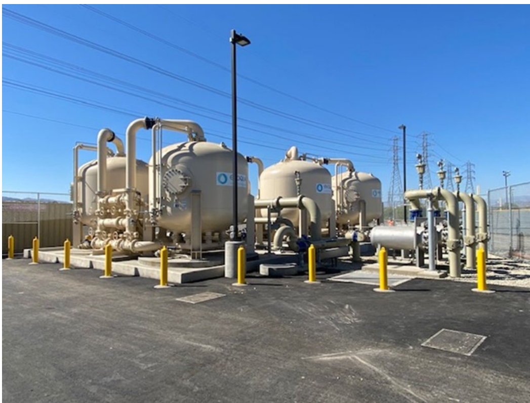
Figure 4: SCVWA N Wells Operating Ion Exchange PFAS treatment system
